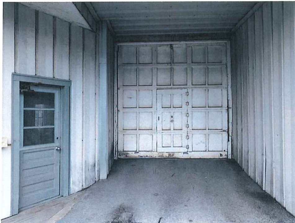
Building #1 – exterior portion of overhead bay door to 2 nd floor ramp (white paint)
