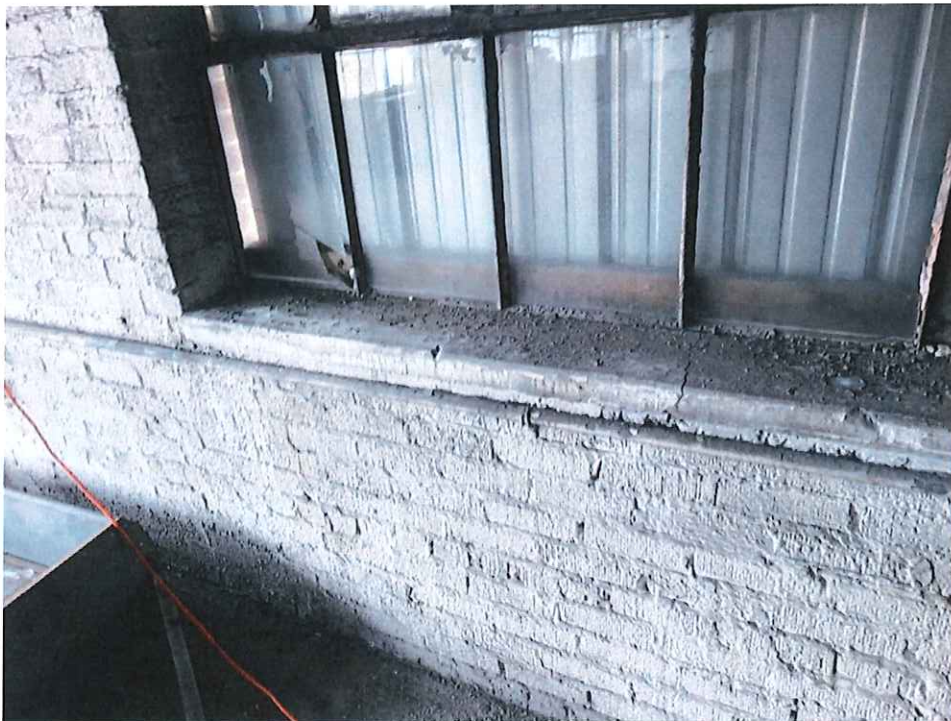
Building #1 – window sills on 2 nd floor (white paint)
